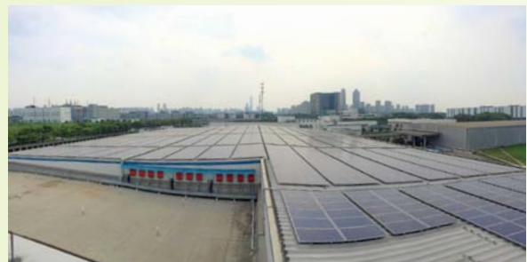
Solar power generation system installed in FUJIFILM Printing Plate (China) Co., Ltd.
