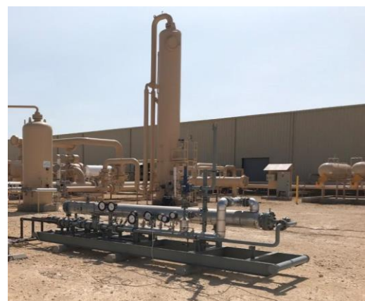
Figure 3: Apura™ FG Skid Installed at the West Texas Compressor Station
